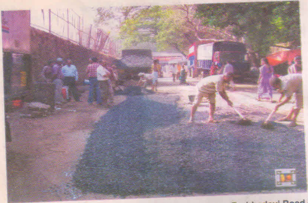
Photo 9- Showing spreading of polymer-Bitumen at New Prabhadevi Road (Opp. Samna Press), Mumbai
